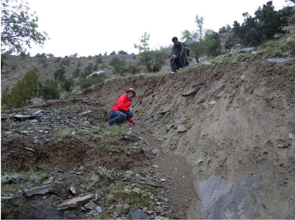
Figure 6: A monitoring moment: measuring the main scarp with a rope. The debris material is sliding over a sloping strata angle as the slope.
