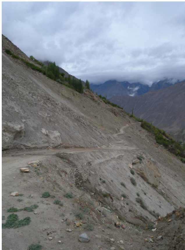
Figure 25: on the way to Holshal, a landslide with a yearly return time.
